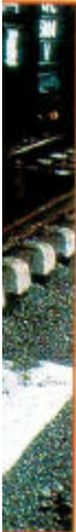
Over a million square metres of Typar geotextile separating barrier were laid on the track during 1998.
