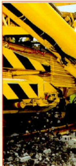
Because of the importance of keeping the track open, removing the track or sleepers is not an option.
