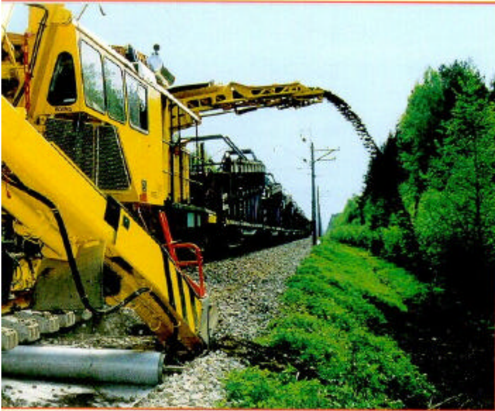
g the line open, a multi-function machine is used to rebuild the railway bed without
